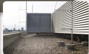
Roof superstructure protected by DEHNiso Combi and DEHNiso roof conductor holder
