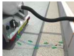
Continuous Ground Loop Monitoring check
