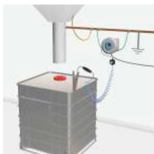
Filling IBCs, Totes, Drums, Containers and Rail Cars
